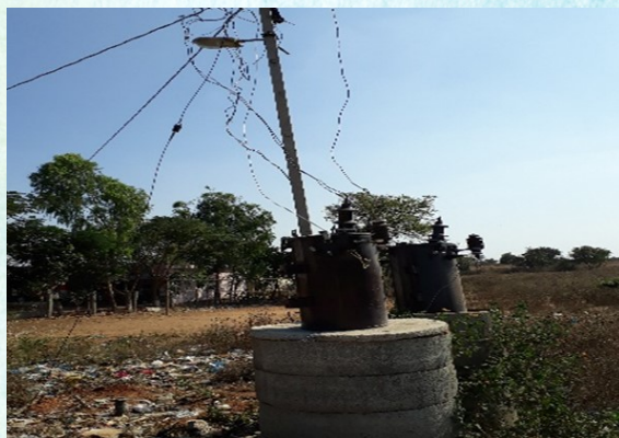
Figure 42: A Transformer at Kadiyala Kunta Tanda
